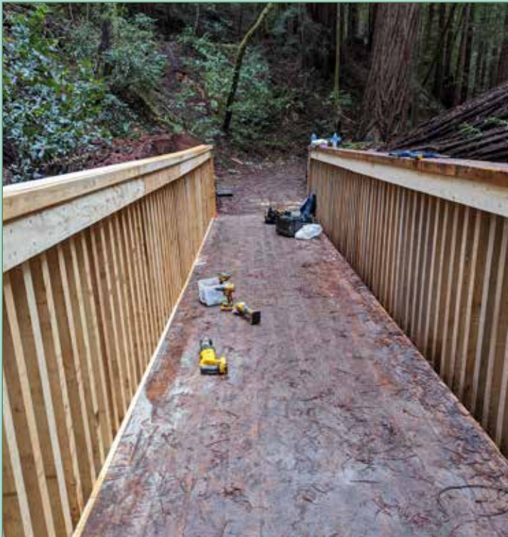
Bridge is done. Thanks to Mike Bushue and his team of volunteers.
